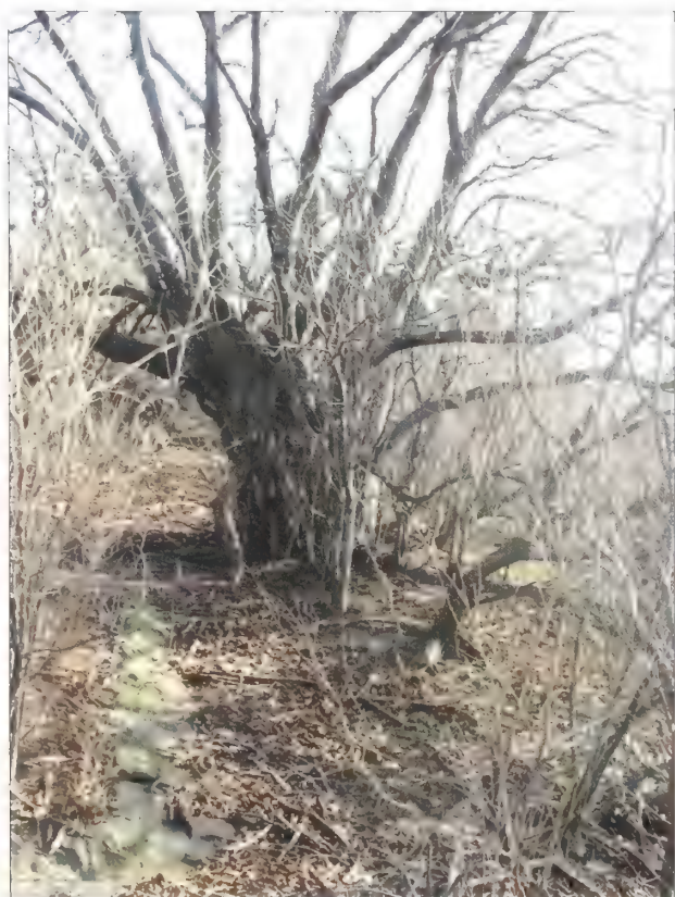
Figure 5.82. View looking south atop of the engineered slope, Battery Kingman. Here, a large tree is seen growing near an exposed concrete feature seen at the left foreground. Woody vegetation should not be permitted to grow on, or within four-feet of concrete battery structures and features (Olmsted Center, January 2009).
